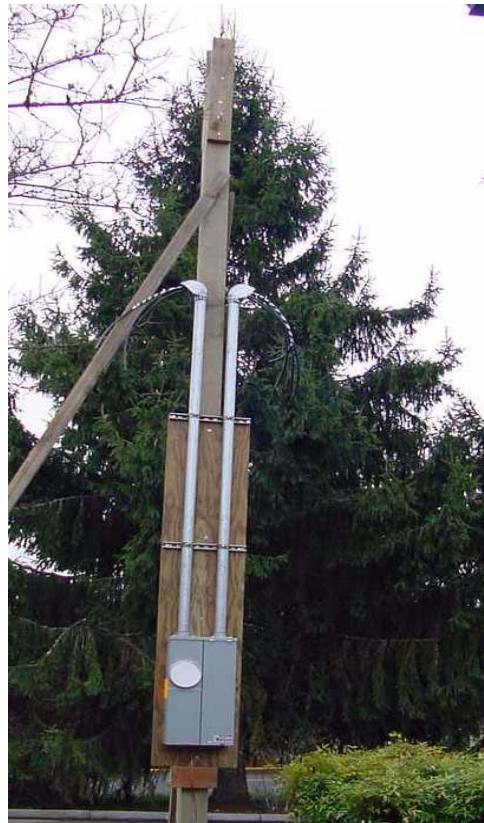
Overhead Temporary Construction Service Poles
