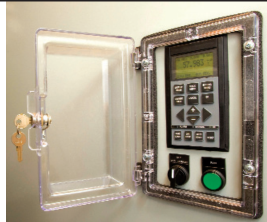
The new VFD computer control adjusts irrigation as needed, saving water and energy.
