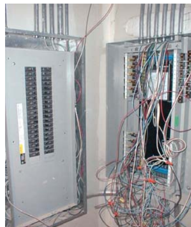
Breaker Box: Controls and regulates the flow of electricity in a house.
