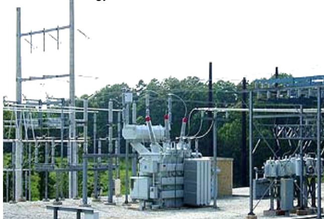
Power Substation: A high-voltage electric facility used to lower or raise voltage, change the type of current, and direct the flow of electricity.
