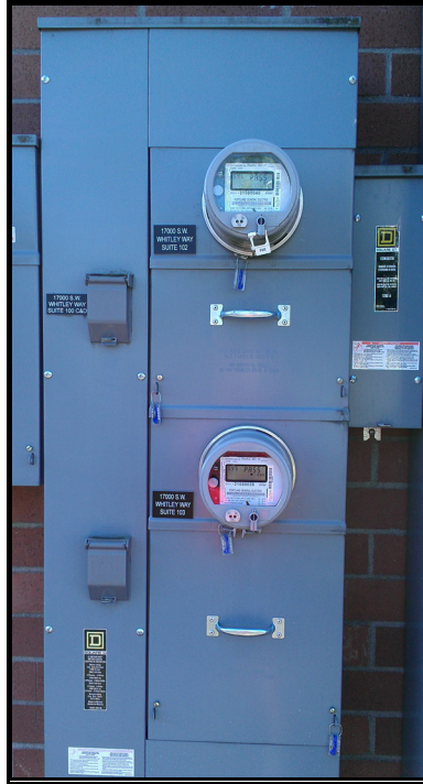
Figure 10-11: Typical Double-Stacked Module Meter Sockets
