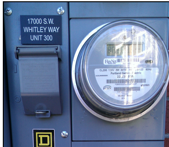
Figure 10-1: Meter Label With Service Address
