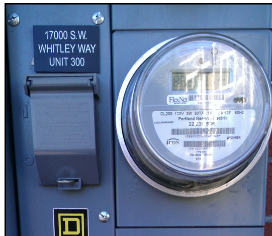
Figure 8-1: Meter Label With Service Address
